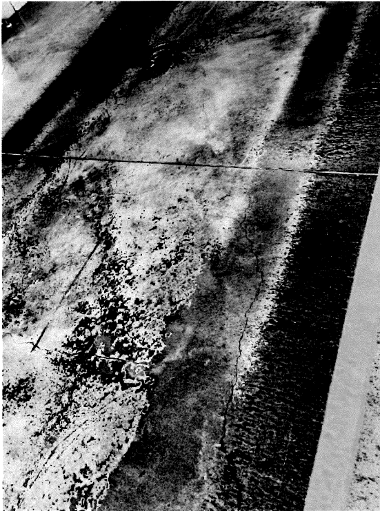
Floor Corrosion and Cracking (Left Bay)
